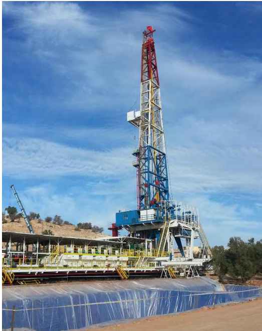
Picture of the 1,500-bhp train-type land drilling rig
