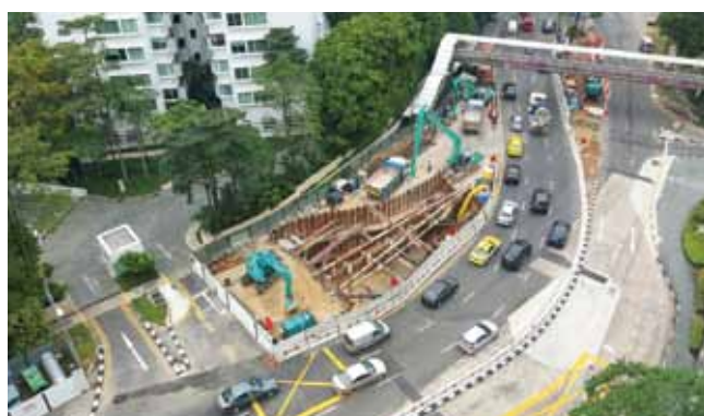
OKP is involved in the construction of Stamford diversion canal – Tanglin and Kim Seng.
