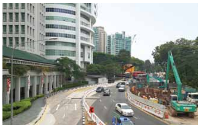
OKP is involved in the construction of Stamford diversion canal – Tanglin and Kim Seng.
