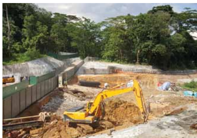
Chye Joo - Or Kim Peow JV is involved in the improvement to Bukit Timah first diversion canal from Holland Road to Clementi Road.
