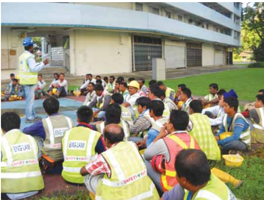
Safety meetings are held regularly at the worksites to ensure occupational health and safety.
