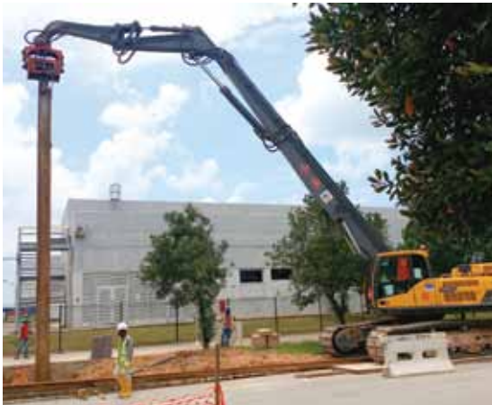
One of our new excavators purchased in 2015 to support our existing projects.
