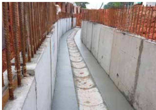
OKP is involved in extension of road, drain and sewer works at Woodlands Avenue 4.
