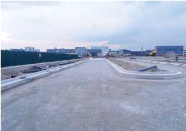
OKP is involved in the construction of roads, drains, sewers and soil improvement works at Tuas South Avenue 7/14.
