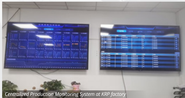
KRP factory located in Kunshan, Jiangsu, China
