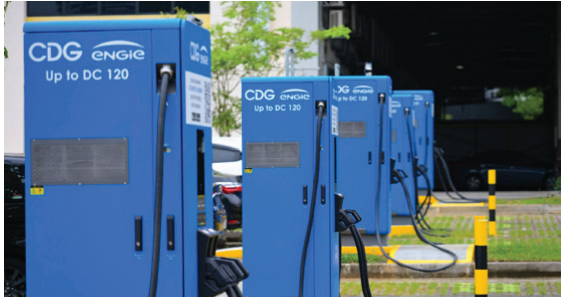
ComfortDelGro ENGIE EV Charging Points at CityCab Building
