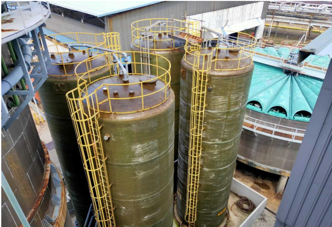
Figure 10: Hydrochloric Acid Storage
