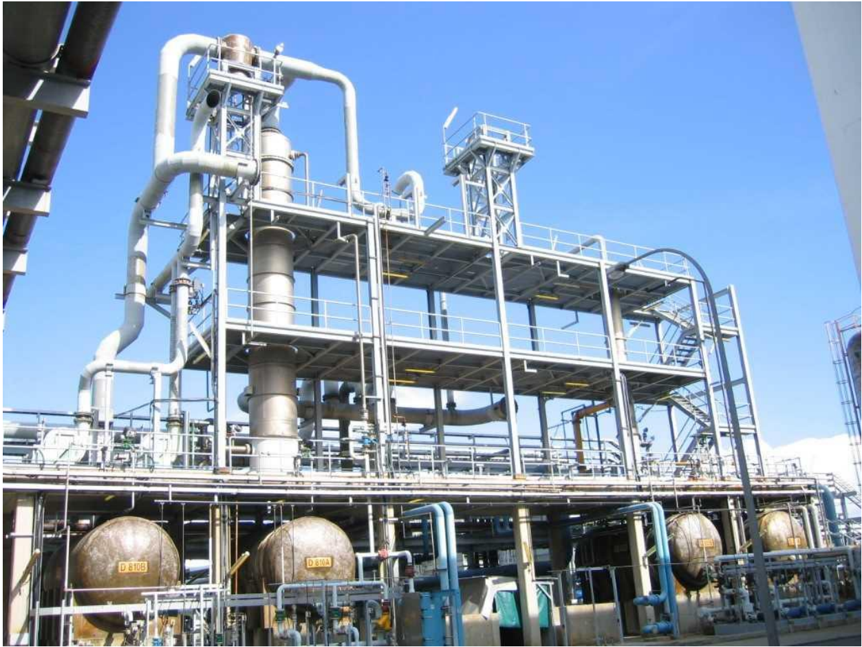
Figure 1: CIL Facility- Sodium Hypochlorite Unit
