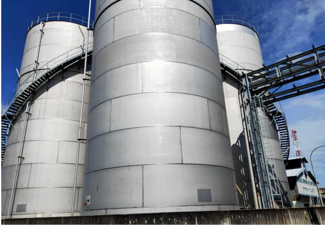
Figure 9: Sodium hydroxide Storage
