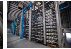
SingSpring Desalination Plant
