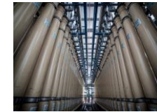
Keppel Seghers Ulu Pandan NEWater Plant
