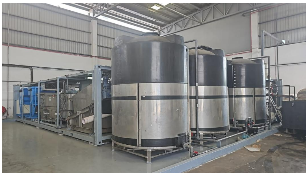
Photo of hazardous waste storage
