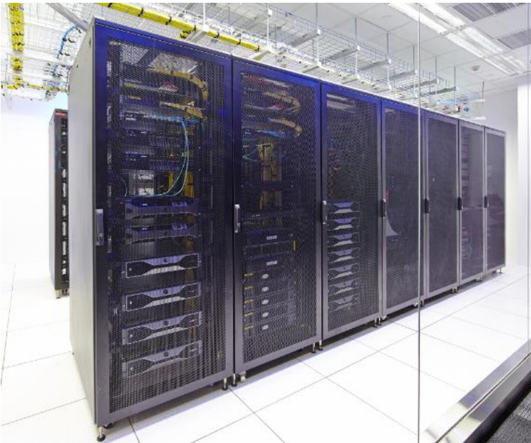
Interior of a data centre facility
