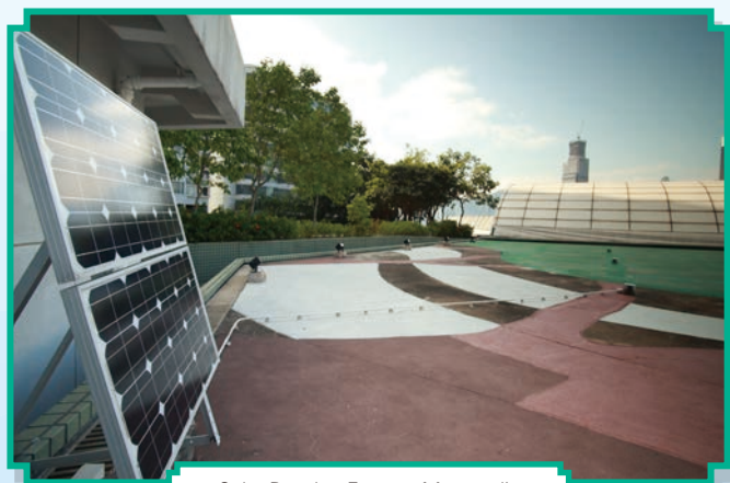
Solar Panel at Fortune Metropolis
