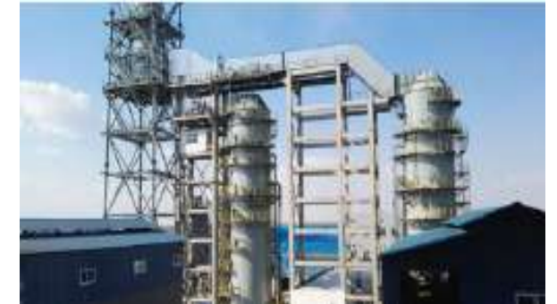
Desulphurization Project of Changrun Project
