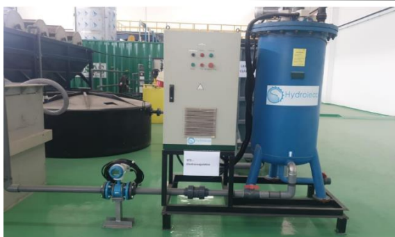
Our WWTP at Kian Teck Facility
