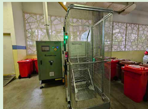
▲ WasteMaster food recycling system testbed at The Robertson House by The Crest Collection
