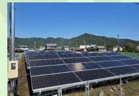
Virtual PPA solar power generation facility installation
