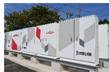
Storage battery system using FORTELION lithium-ion secondary batteries (Kanazu Murata Manufacturing)
