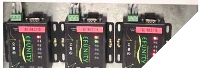
Installed sub-sensors to enable a more precise monitoring of energy consumption at SETSCO's premise.
