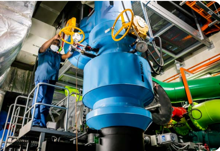
High-efficiency District Cooling Plant in RWS
