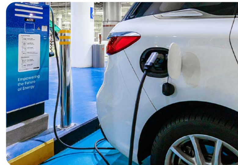
An EV charger in operation at our carpark
