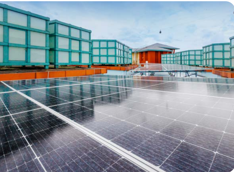
New solar panels installed at Hard Rock Hotel Singapore
