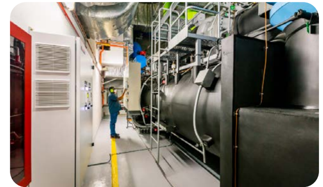
District Cooling Plant Operations
