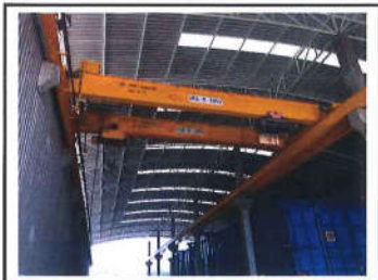
OVERHEAD CRANE 5 TONS BLAST 02-PM-000032, 000033
