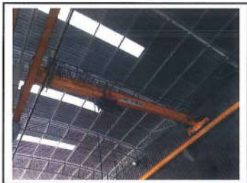
ELECTRIC WIRE ROPE HOIST FOR OVERHEAD CRANE 5 TONS 02-PM-000031
