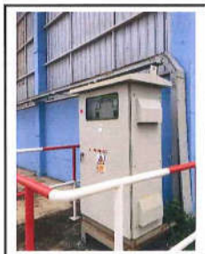
TRANSFORMER 250 KVA. ELECTRIC SUB STATION
