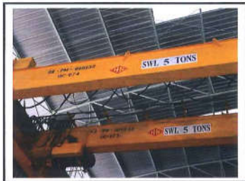
OVERHEAD CRANE 5 TONS BLAST 02-PM-000032, 000033
