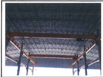
OVERHEAD CRANE 5 TONS SHOP 1 - OC-055
