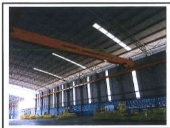
OVERHEAD CRANE 5 TONS SHOP 2 - OC-068
