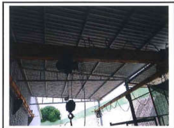
OVERHEAD CRANE CAPACITY 2 TONS 01-PM-0603
