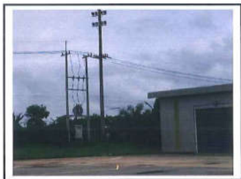
TRANSFORMER 250 KVA (02-PM-000277)
