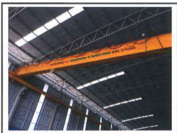
OVERHEAD CRANE 5 TONS SHOP 2 - OC-062
