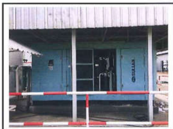
AIR COMPRESSOR SULLAIR 24KT LS25S-350 LACKT[RUN 30/5/2011] (02-PM-000007)
