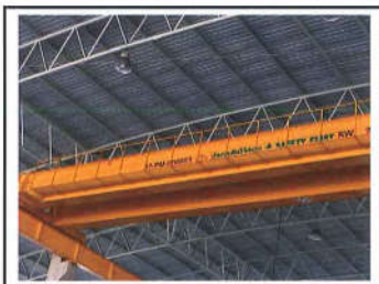
OVERHEAD CRANE 20 TONS C/W STRUCTURE SHOP 1 - OC-057
