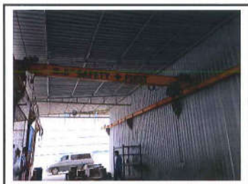
OVERHEAD CRANE 2 TONS PAINT SHOP 01-PM-0618
