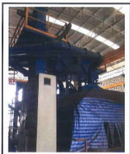
AUTOMATIC SHOT BLAST MACHINE 02-PM-000167
