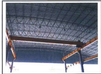
OVERHEAD CRANE 5 TONS SHOP 1 - OC-054
