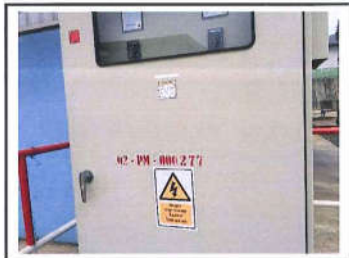
TRANSFORMER 250 KVA. ELECTRIC SUB STATION
