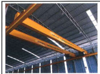
OVERHEAD CRANE 5 TONS SHOP 1 - OC-059
