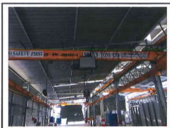
OVERHEAD CRANE SINGLE FRIDER 7.6M. HOOK EBN-030 LN 3 TONS
