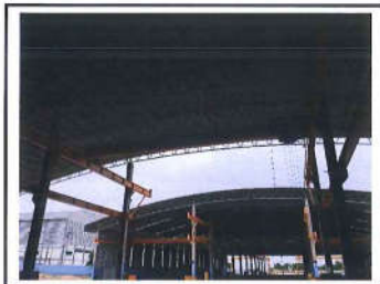
OVERHEAD CRANE 5 TONS SHOP 2 - OC-052
