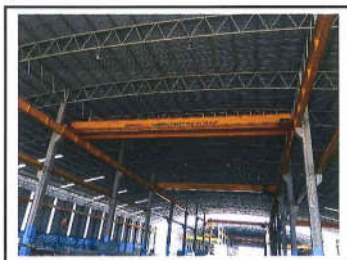
OVERHEAD CRANE 10 TONS SHOP 2 - OC-066
