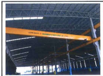
OVERHEAD CRANE 5 TONS SHOP 1 - OC-050
