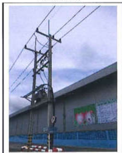
TRANSFORMER 250 KVA (02-PM-000005)
