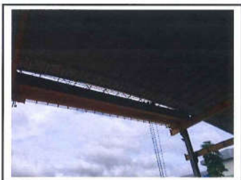
OVERHEAD CRANE 10 TONS SHOP 2 - OC-067
