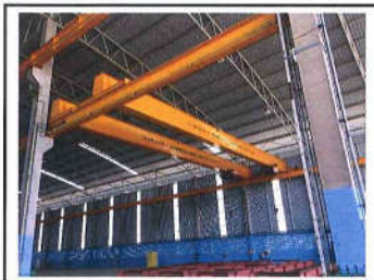
OVERHEAD CRANE 5 TONS SHOP 1 - OC-058
