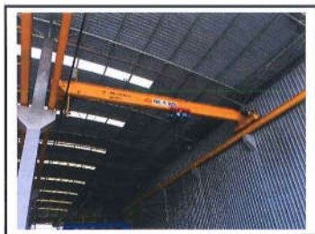
ELECTRIC WIRE ROPE HOIST FOR OVERHEAD CRANE 5 TONS 02-PM-000030
