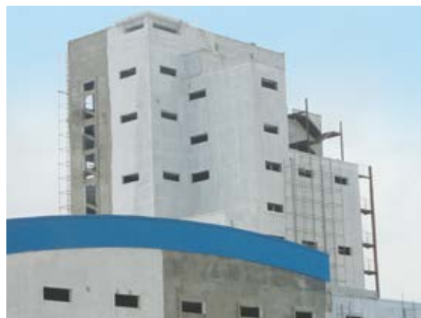
Spray Dried Coffee Tower in Andhra Pradesh, India
