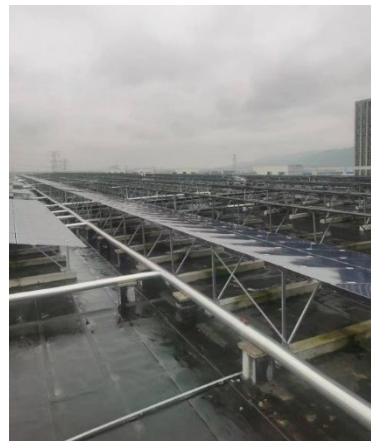
Solar panels at the Fuzhou E-commerce property
