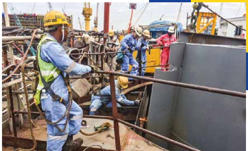
Above: Safety harnesses is a must for workers when working in height on-board vessels.
