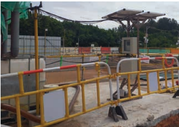
Use of Solar Panels for TSS Reader at site
