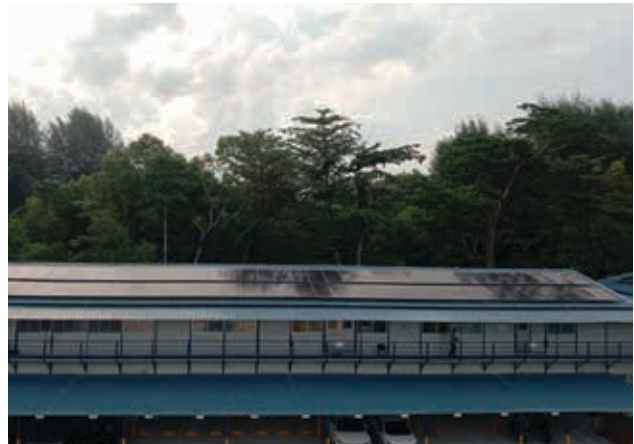
Rooftop solar panels for site office
