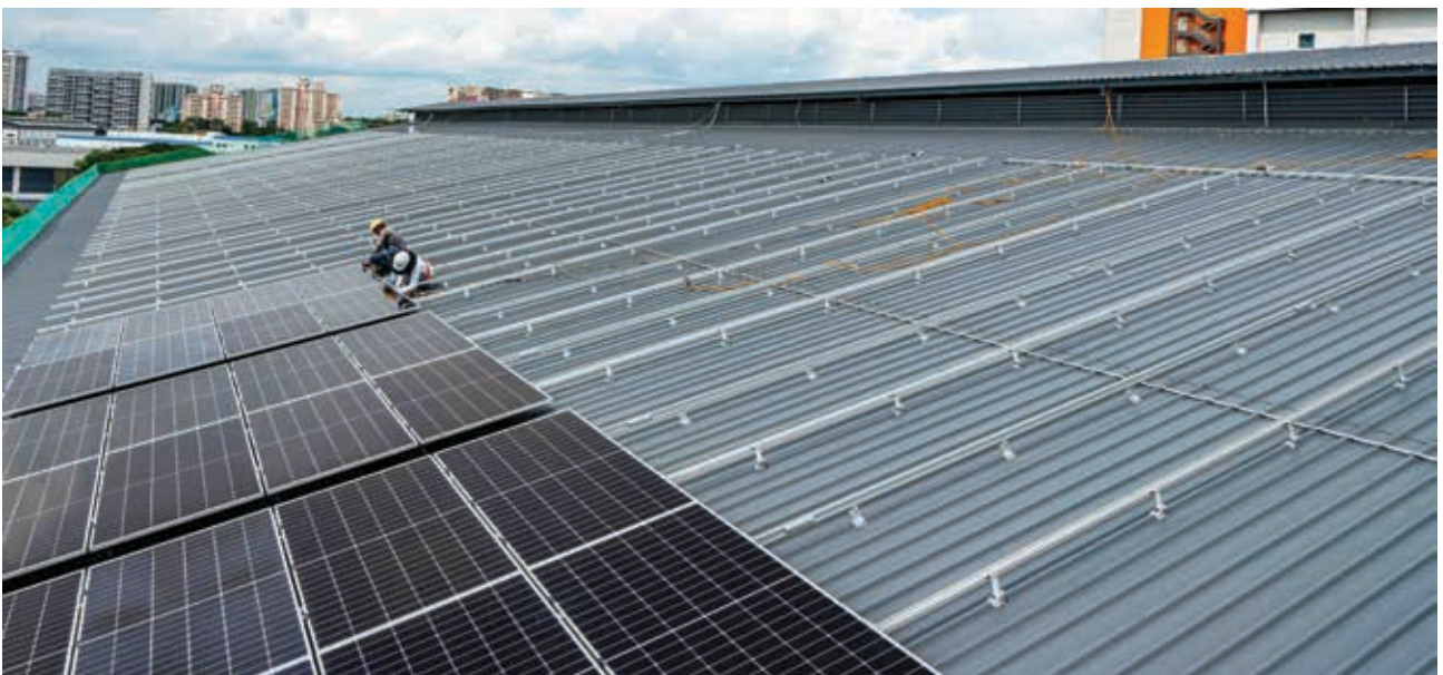
Figure 2: Solar panels being installed on West facing roof of Chin Bee Factory. West and East facing roofs will be installed with solar panels, covering a total area of 4,008 m 2 . Works will be completed in February 2023, providing 6.1 million kWh of solar energy to Chin Bee factory for the next 12 years.
