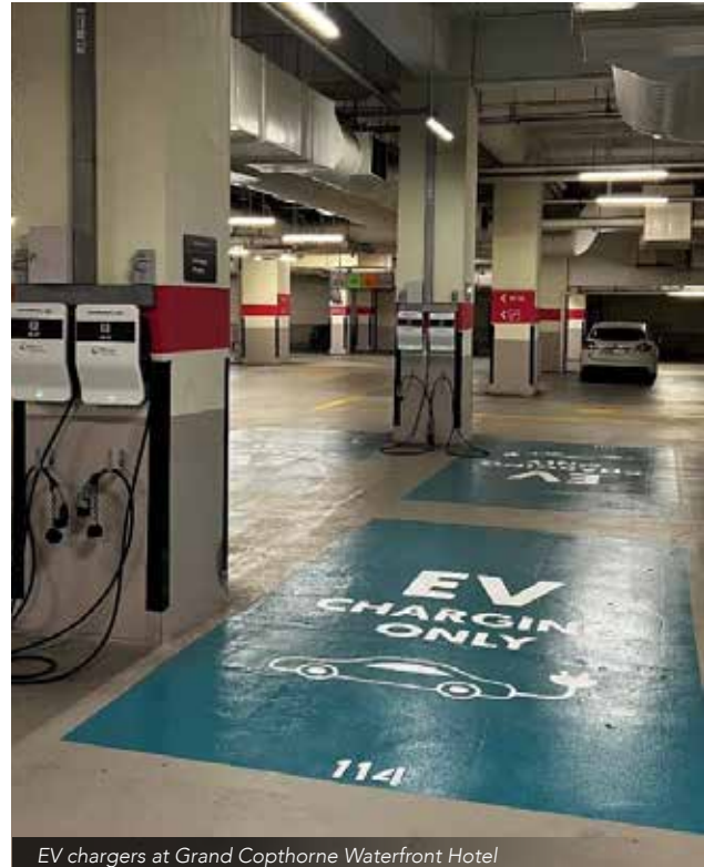
EV chargers at Grand Copthorne Waterfront Hotel
