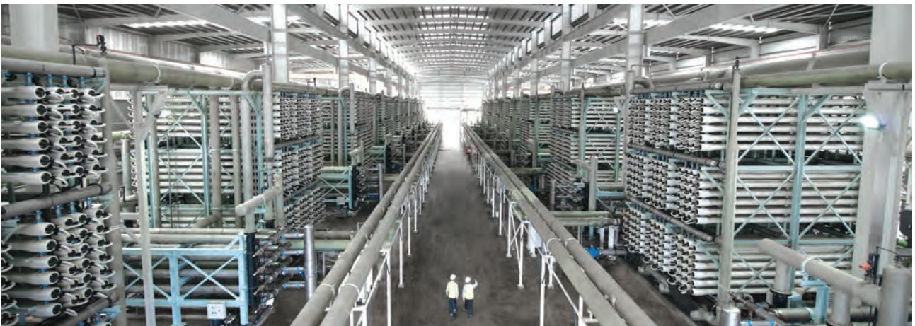
Hyflux's Tuaspring IWPP in Singapore, is the only integrated water and power project in Asia
