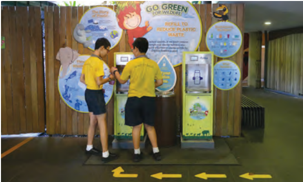
Water dispensers designed and installed by Hyflux at WRS parks
