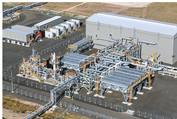
Condabri North Gas Processing Facility
