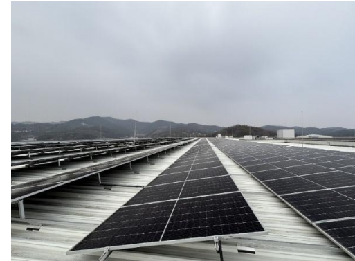
South Korea | Anseong Logistics Centre Solar capacity: 998 kW
