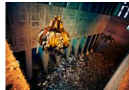
Keppel Seghers Tuas WTE Plant
