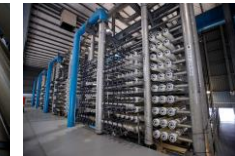
SingSpring Desalination Plant
