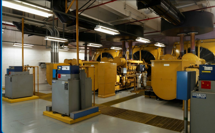
Prime-Rated Generators Support Resiliency
