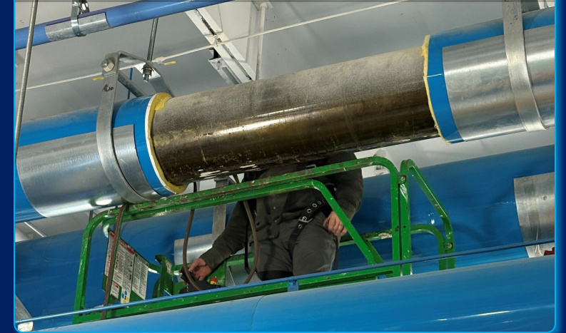
Enhanced Chiller Plant Efficiency
