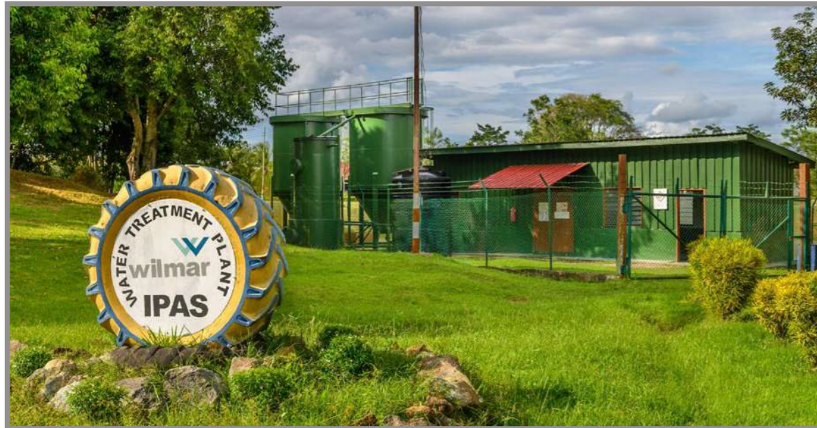
Water treatment plant in Wilmar's Sapi Plantation, Sabah
