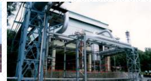
Flare Gas Recovery, ONGC, Uran
