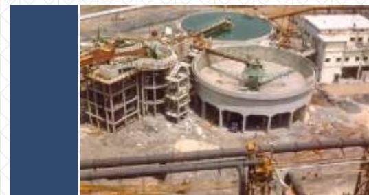
WWTP & Recirculation Plant for LD-2 Tata Steel, Jamshedpur
