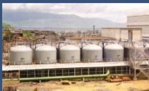
High Rate Filtration Plant for Hot Strip Mill - TISCO, Jamshedpur
