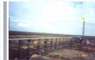
Gas Lift Facilities for GGS-IV, ONGC Pakhajan
