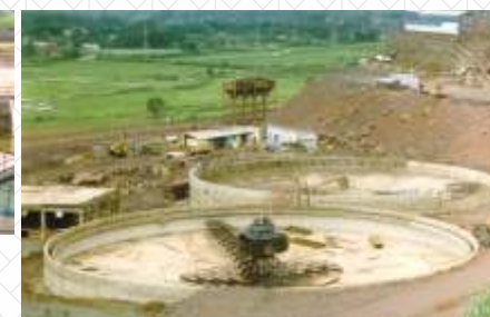
WWTP & Recirculation plant Tata Steel, Joda
