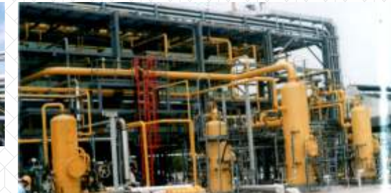
HP Gas Compression Plant – ONGC, Geleki
