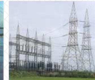
Cabling for 400kV Sub-station NHPC, Jeypore
