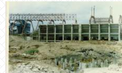
Raw Coal Bunker – Tata Steel, West Bokaro
