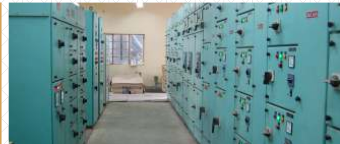
Electrical Control Room of Gas Condensation Plant – SAIL, Burnpur
