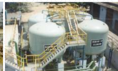
High Rate Filtration Plant for Rebar Mill - Tata Steel, Jamshedpur
