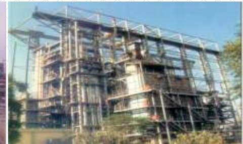
Ammonia Water Front End Plant – Heavy Water Board, Vadodara
