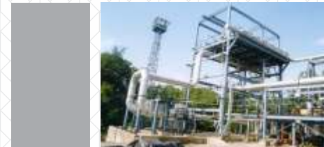
HUT-BUT Oil Line & Methanol Injection Facilities, ONGC, Uran
