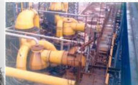
Final Gas Cooler & Naphthalene Scrubber Plant – Konark Metcoke
