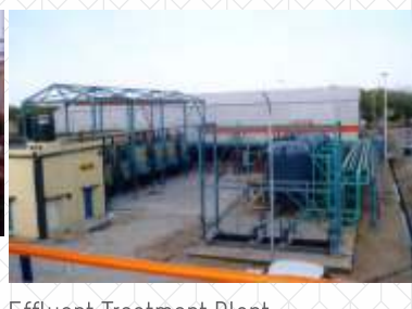
Effluent Treatment Plant ONGC, North Kadi
