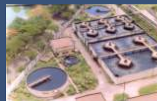
Biological Oxidation Plant, SAIL Rourkela
