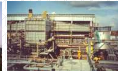
Hydrogen Reformer Pkg Indian Oil, Barauni Refinery
