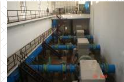
Booster Pumping Station at Kalighat Park – IRCON, Kolkata
