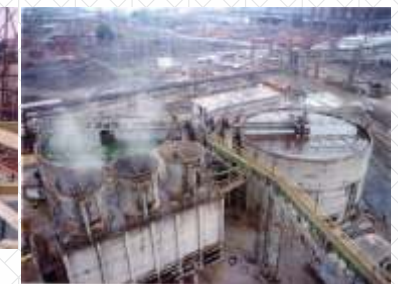
Water Circulation System for LD-1 Tata Steel, Jamshedpur
