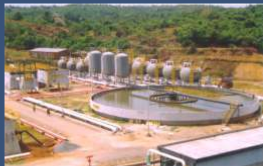
Waste Water Treatment Plant, Mangalore Refineries & Petrochemicals Limited
