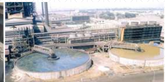
Dirty Water Treatment & Recirculation Plant JSW, Bellary
