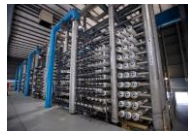
SingSpring Desalination Plant
