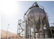
Aramco Gas Pipelines Company
