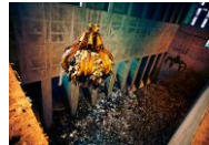
Keppel Seghers Tuas WTE Plant
