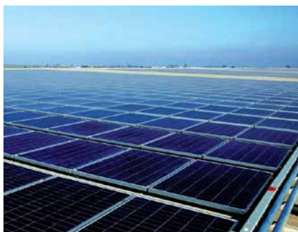
Solar panels in our Hanford tomato production facility
