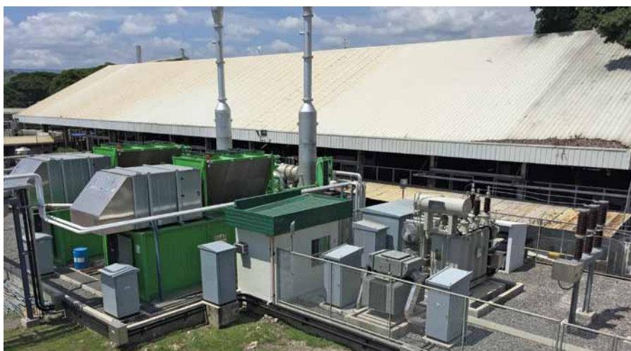
The generator sets for the waste-to-energy facility
