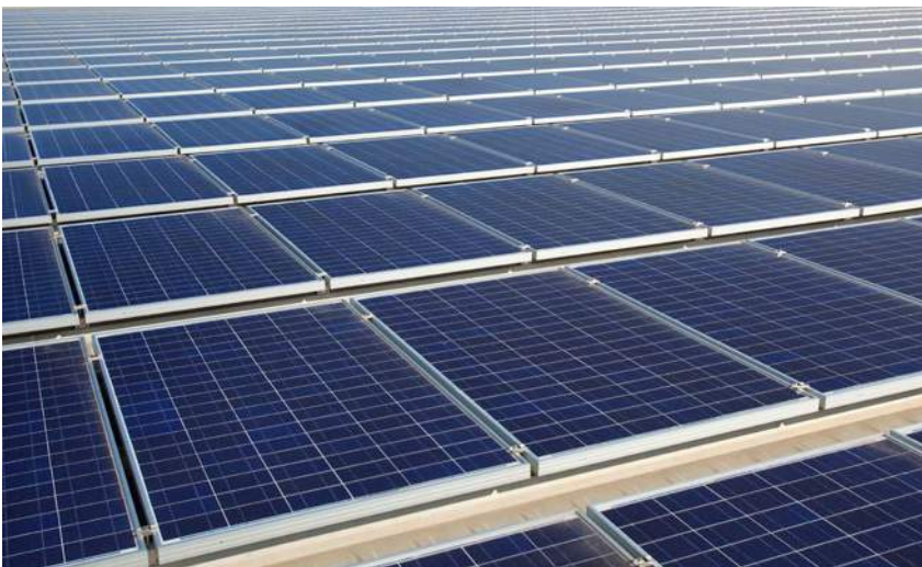
Solar panels in Hanford facility in California, USA
