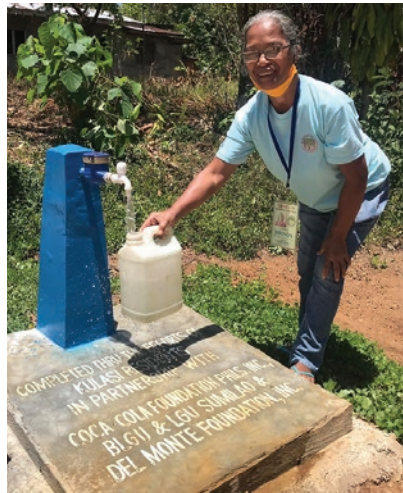
Water system installed in a locality in Bukidnon
