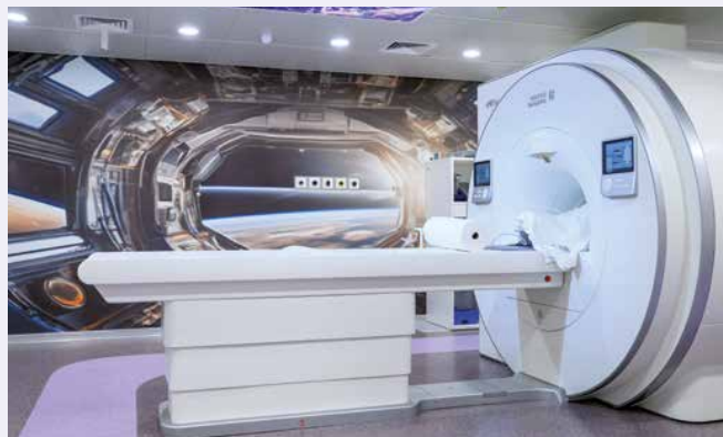
The installation of a state-of-the-art 3 Tesla (“3T”) MRI machine has significantly advanced our diagnostic imaging capabilities.
