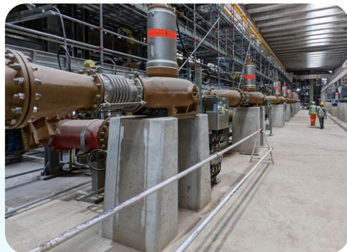
Membrane gallery of Changi WRP Phase 2.
