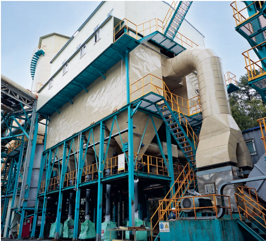
EMK operates the third largest number of WTE plants with a combined incineration capacity of 419 tonnes per day.
