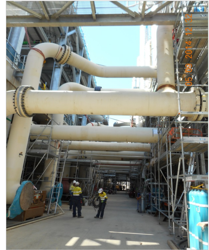
Pipe connections between Compressor Building and Module 101D (Cryo Coolers)
