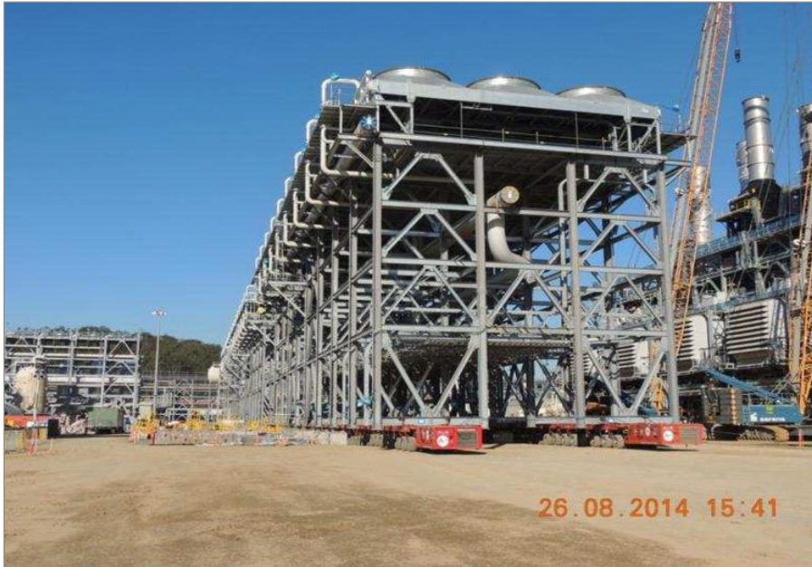
Setting Module 202NB (Propane Condenser)
