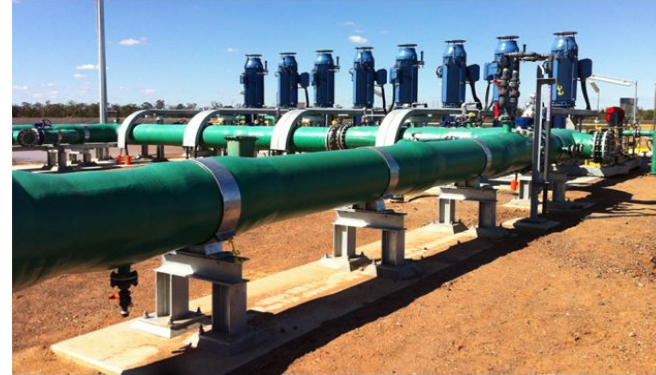
Condabri Central – Feed Pump Station
