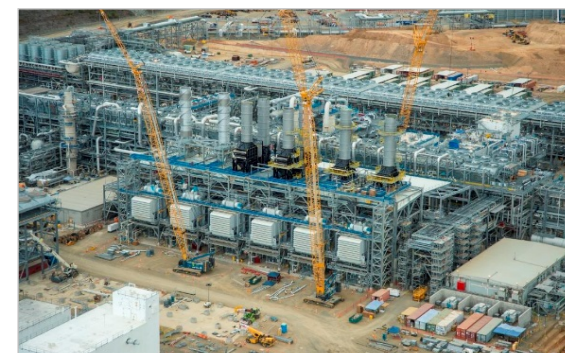
Overview of Train 1 Inside Battery Limits (ISBL)
