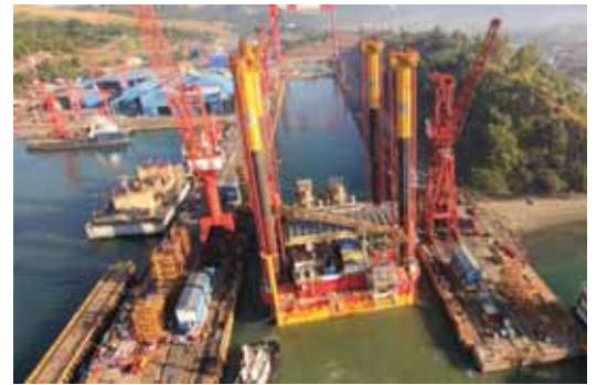
Shell's Depletion Compression Platform
