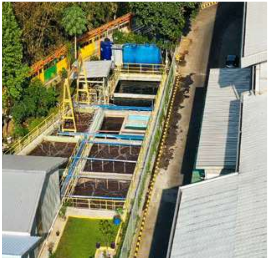
IPAL di SGF Boyolali WWTP at SGF Boyolali
