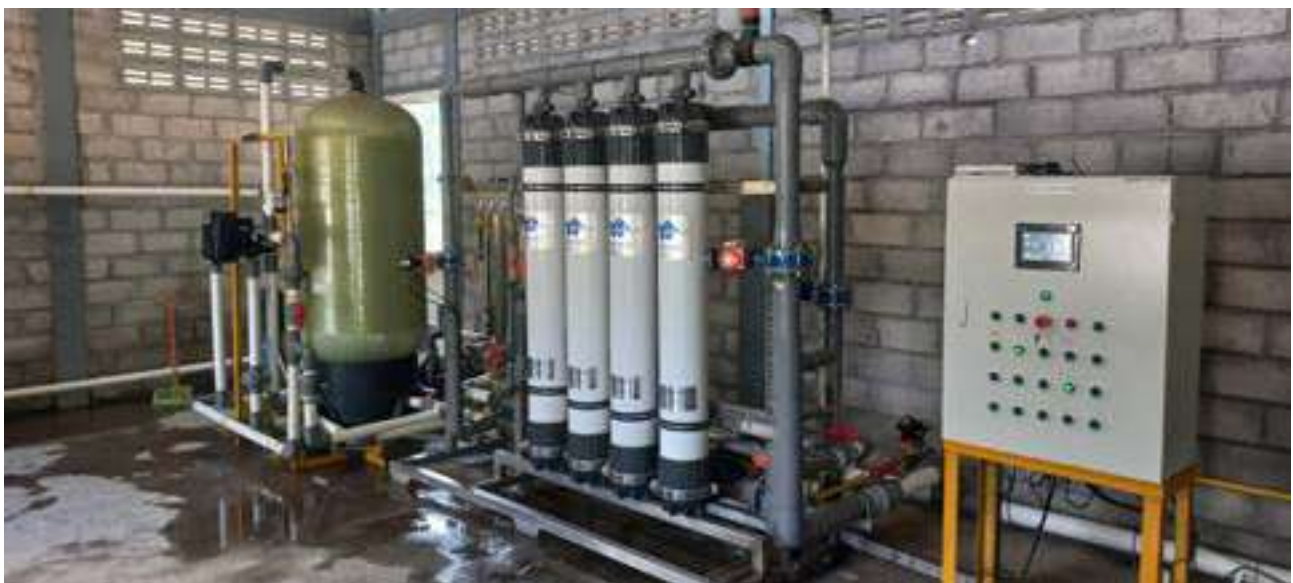
Fasilitas Daur Ulang Air Wastewater Recycling Facility
