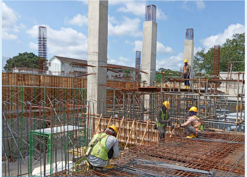
Ongoing Projects at Johor River Waterworks NEW DISINFECTION SYSTEMS
