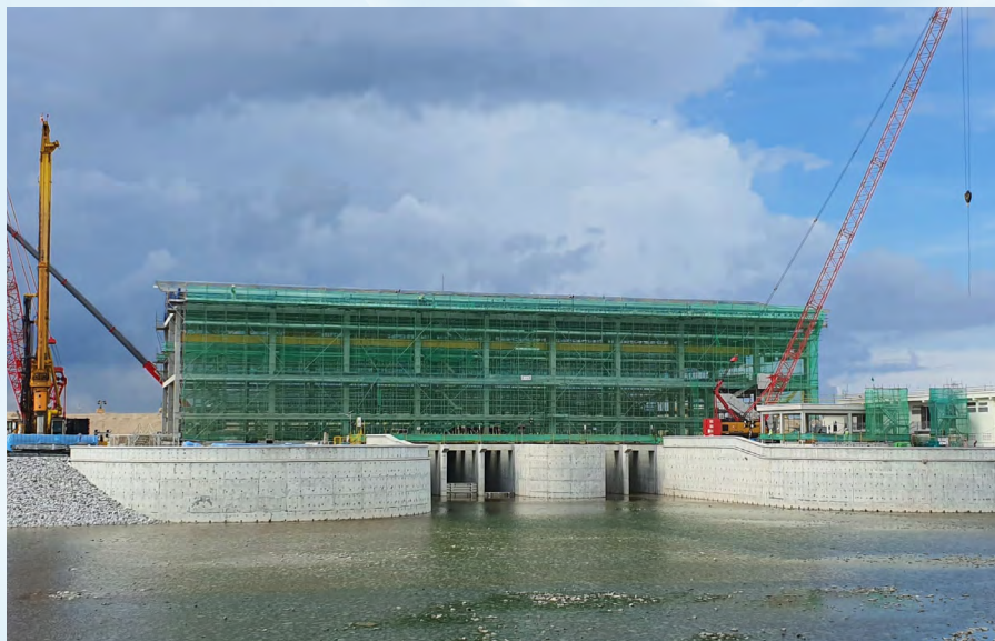
Ongoing Projects at Pulau Tekong SUPPLY AND INSTALLATION OF MECHANICAL PACKAGE WORKS FOR THE CONSTRUCTION OF POLDER
