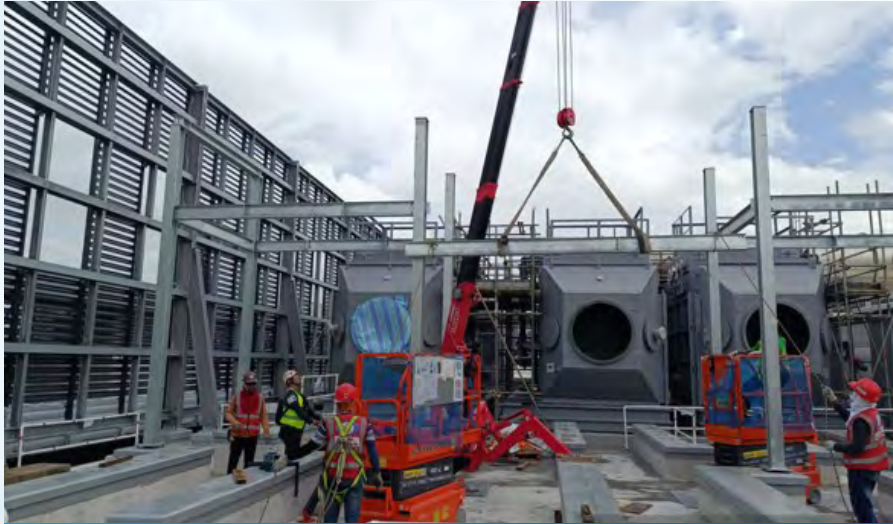
Ongoing Projects for Enviro Plant & Engineering Pte Ltd INSTALLATION OF PROCESS EXHAUST SYSTEM AT UMC
