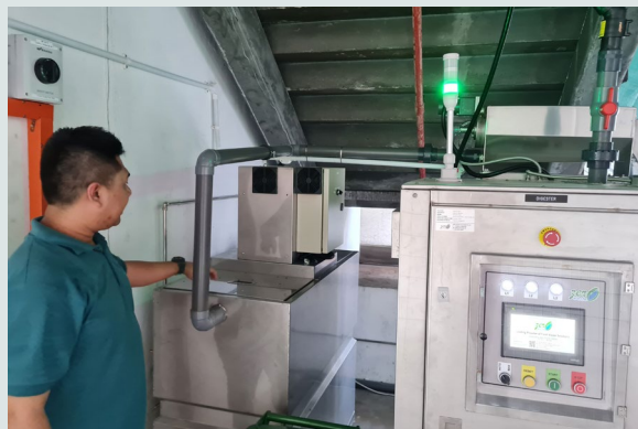
The supplier of the food waste digester explained how the machine works to convert food waste into discharge as greywater.
