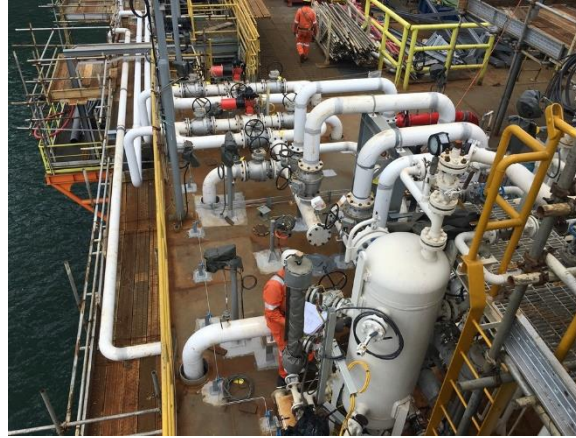
Process pipework on Ingenium II deck
