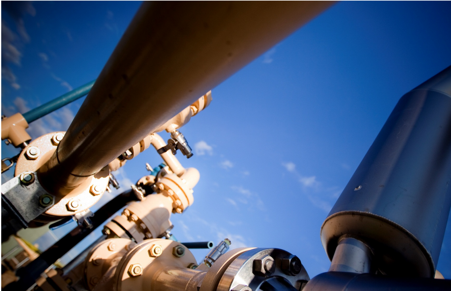
Pressure reduction station
