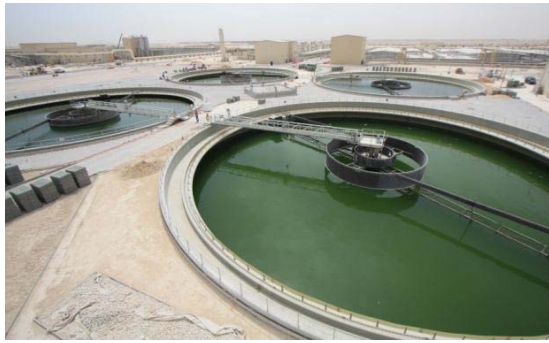
Doha North Sewage Treatment Works, Qatar
