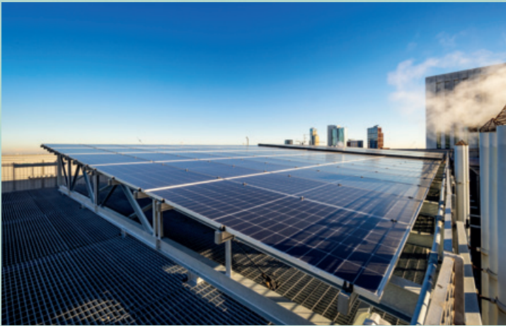
Photovoltaics (PV) panels on Ropemaker's rooftop provides solar energy into the building which is used in the common areas, keeping electricity supply costs down. In 2023, the PV output has increased by 155% as a result of the additional PV panels installed.
