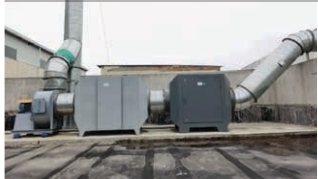
FYSZ – Exhaust Gas Treatment System for Oil Mixing Room and Hazardous Waste Warehouse (completed in 2019)
