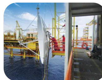
Deployment of telecommunications systems by O'Connor's
