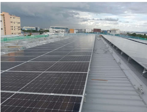
FYC - Solar panels
