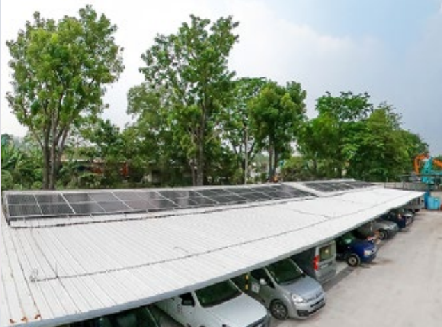
Solar panels at Jalan Papan project site office.
