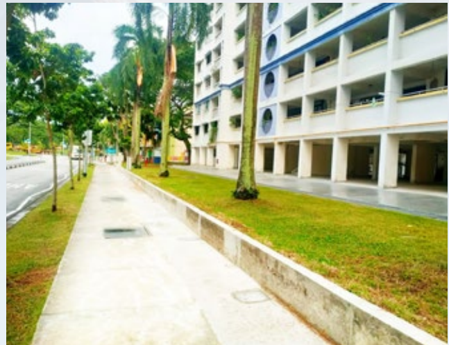
Completed work using CMC for Commuter infrastructure Enhancement project along Kampong Arang Road.
