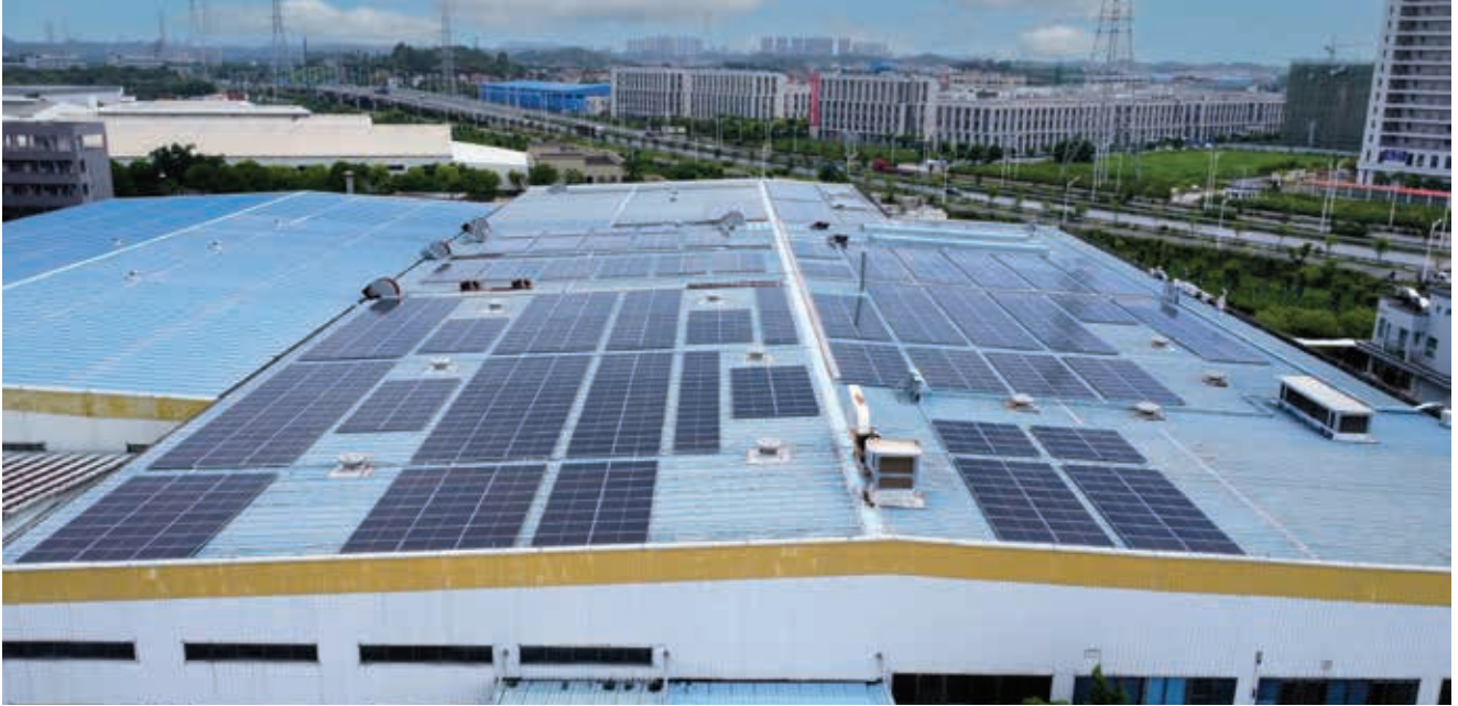
Solar Photovoltaic Panels in China Guangzhou Plant
