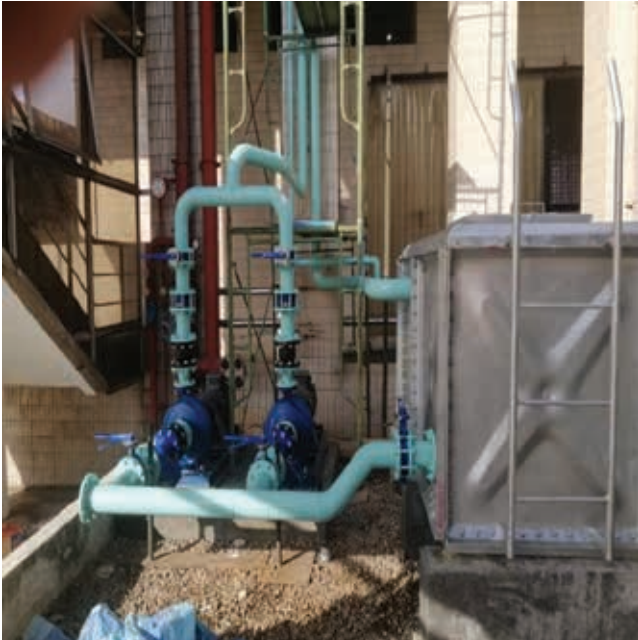
New Hydromatic Cooling Tower in Johor Bahru Plant
