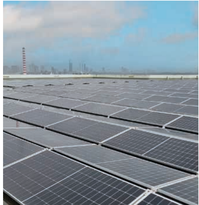
Solar Photovoltaic Panels in Singapore Senoko Plant
